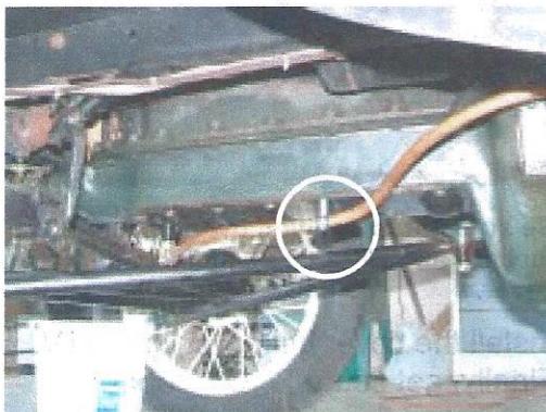
Here, I used a small bushing and a rubber lined clamp. You really need to isolate this line from vibrating. Copper has a nasty habit of breaking when allowed to vibrate.
