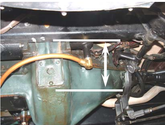
Marked on the above photo are the collection and delivery levels. The total drop is 4 \frac{3}{4} inches, which is steeper than the Ford internal oil line. This line should still deliver oil
