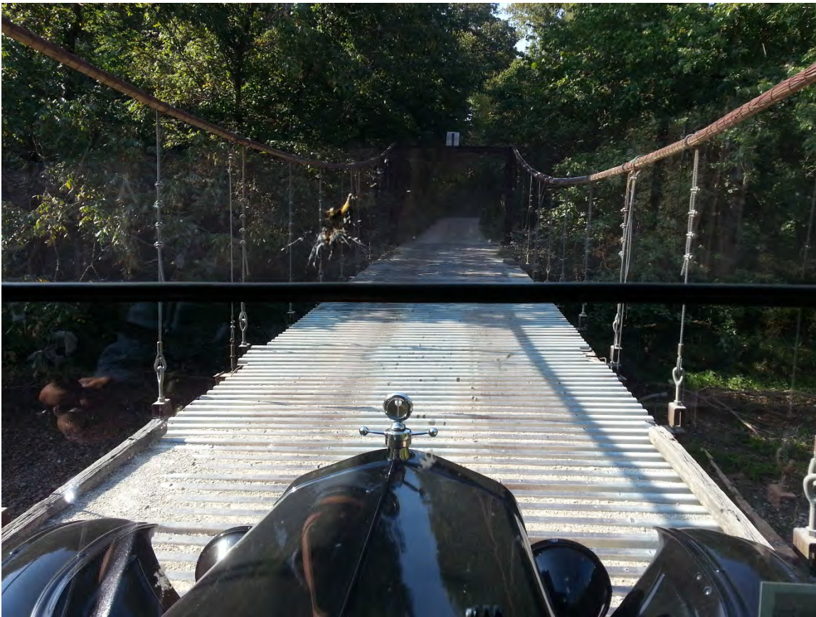
BRIDGE IS SWAYING (and CREAKING and GROWLING)... NOTE: the sand filled roadway DID NOT soften the ride!
