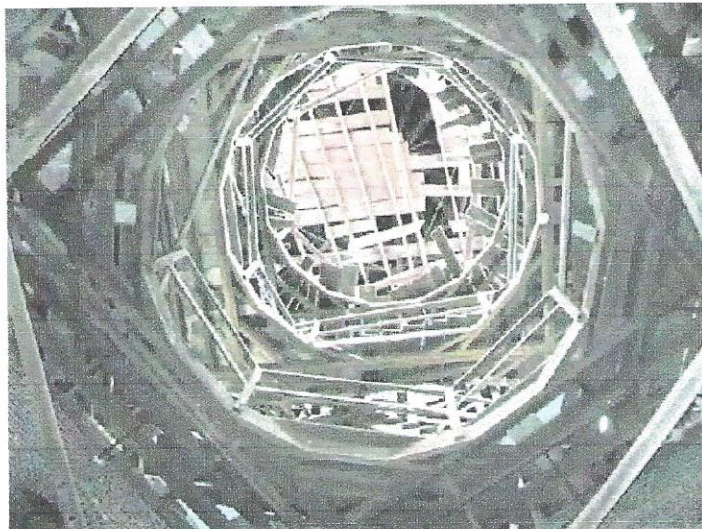
Standing in the middle of the first floor, looking up at the unfinished upper floors.
